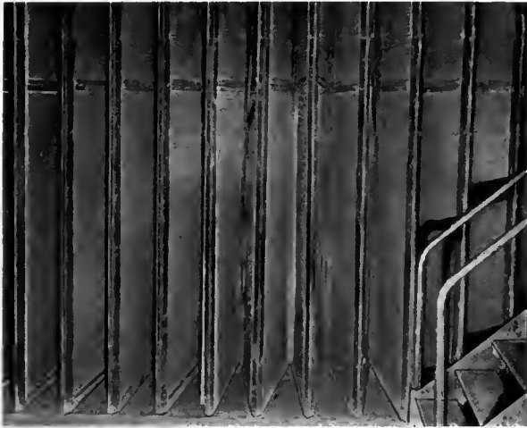
A SECTION OF ONE OF THE AIR FILTERS
